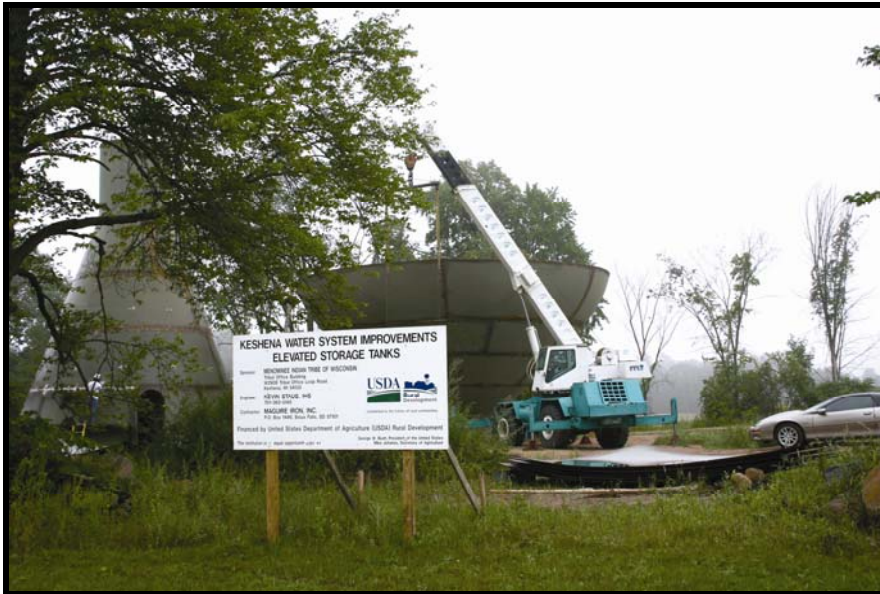
The Tribal Utilities Department unveiling the Keshena System Improvements Elevated Storage Tanks, photo courtesy of Menominee Nation News.
